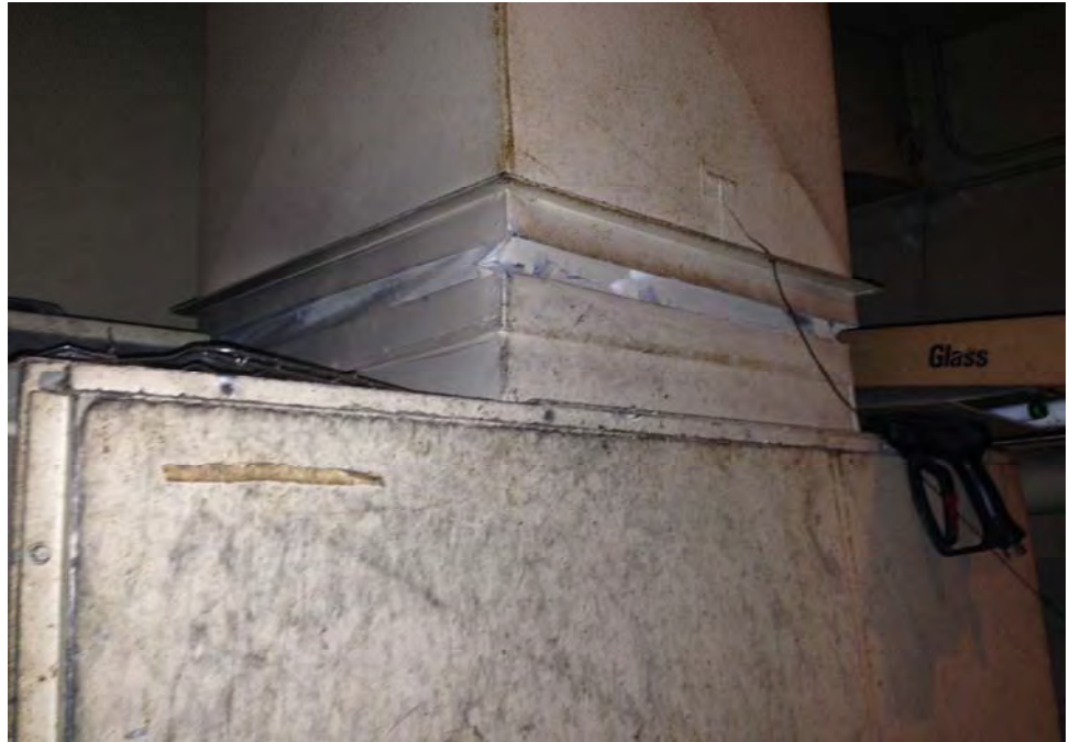
Photograph 9: View of assumed asbestos containing vibration damper in the mechanical room of the restaurant building.
