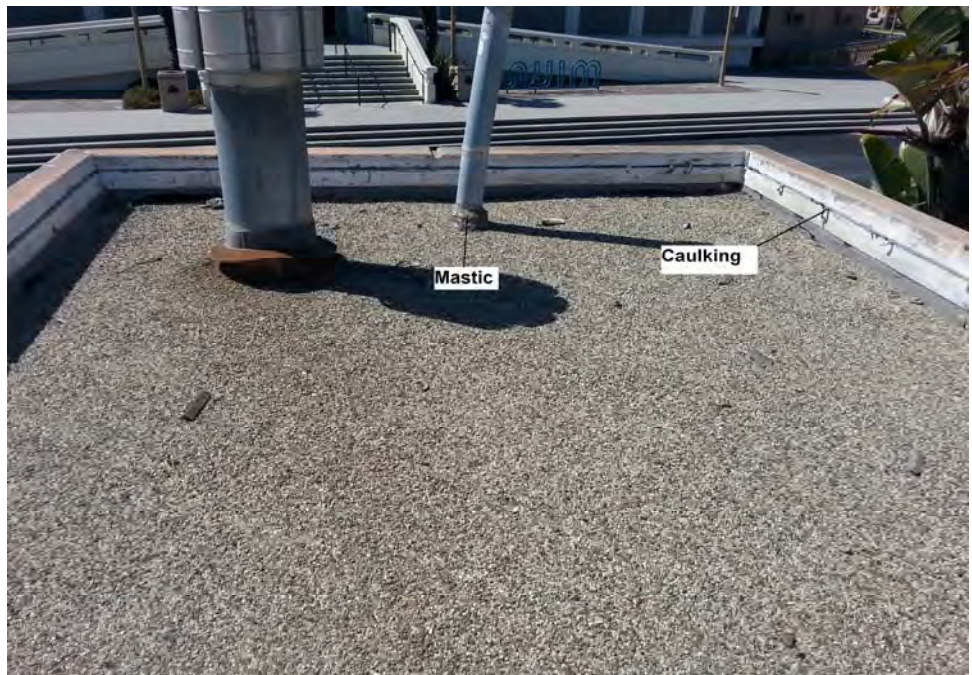
Photograph 10: View of old pool mechanical/chemical building roofing with asbestos containing materials including vent black mastic and gray caulking.
