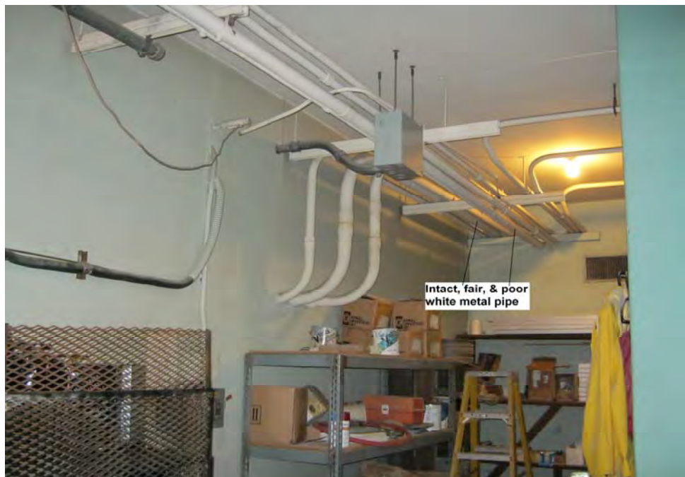
Photograph 22: View of representative intact, fair, and poor lead-containing white paint on metal ceiling pipes in the pool equipment storage room in the basement of the main pool building.
