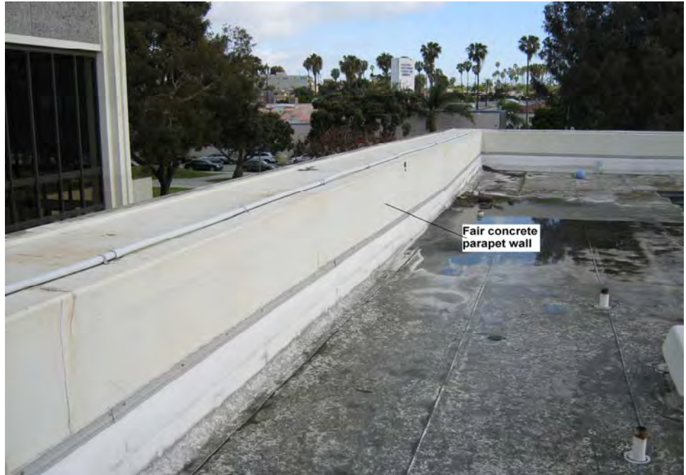
Photograph 25: View of fair lead-containing white paint on concrete parapet wall on the roof of the locker rooms and office building.
