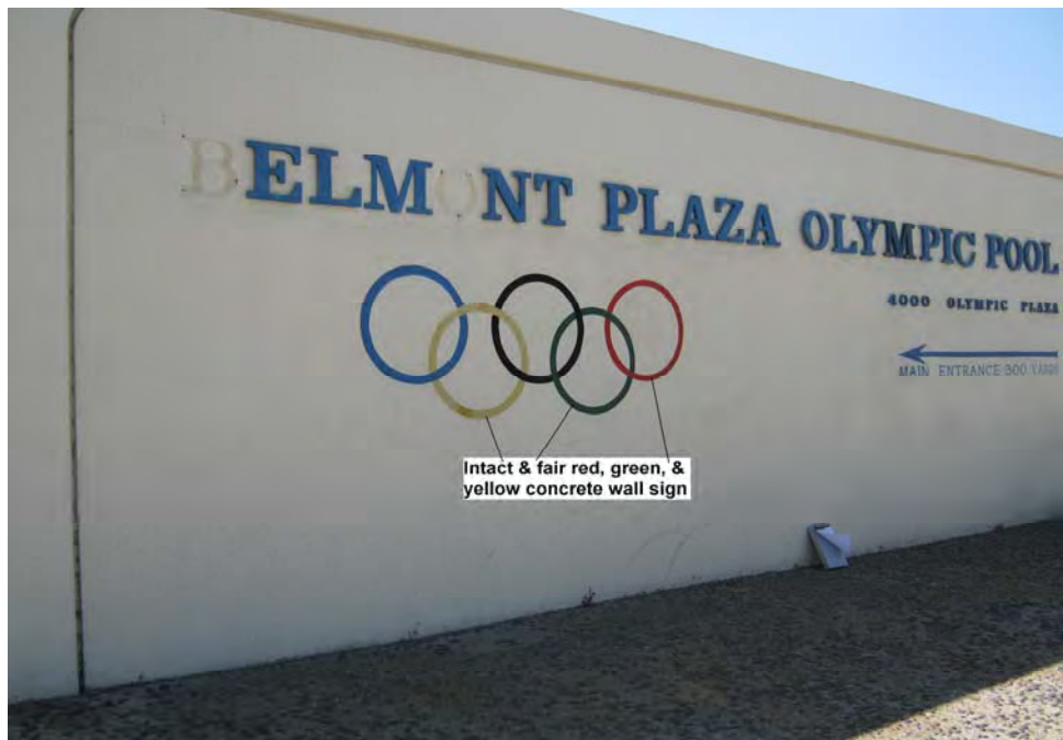
Photograph 16: View of intact and fair lead-containing red, green, and yellow paint on concrete wall sign on the exterior wall of the ramp.
