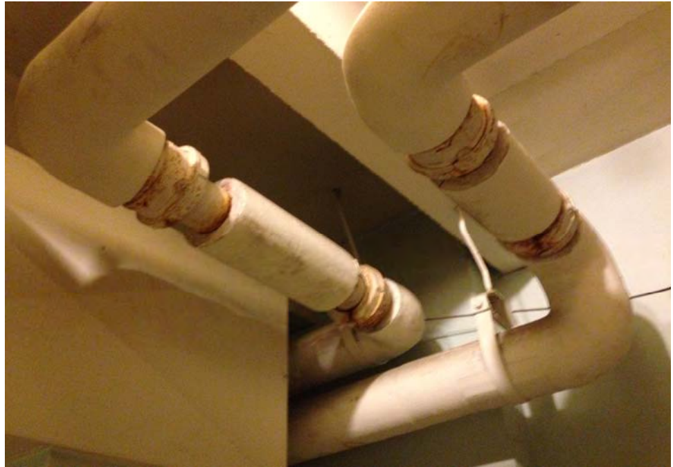
Photograph 5: View of representative asbestos containing cloth-wrapped elbow insulation in the main pool building basement.
