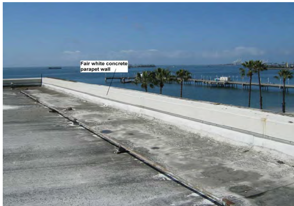
Photograph 18: View of fair lead-containing white paint on concrete parapet wall on the roof of the main pool building.
