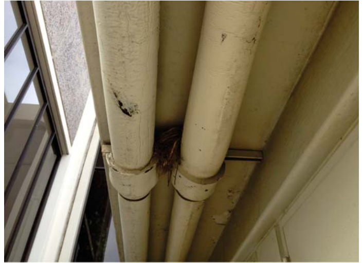
2. One nest observed on top of pipes that run under Del Mar Room ramp, but no birds observed occupying or visiting the nest.
