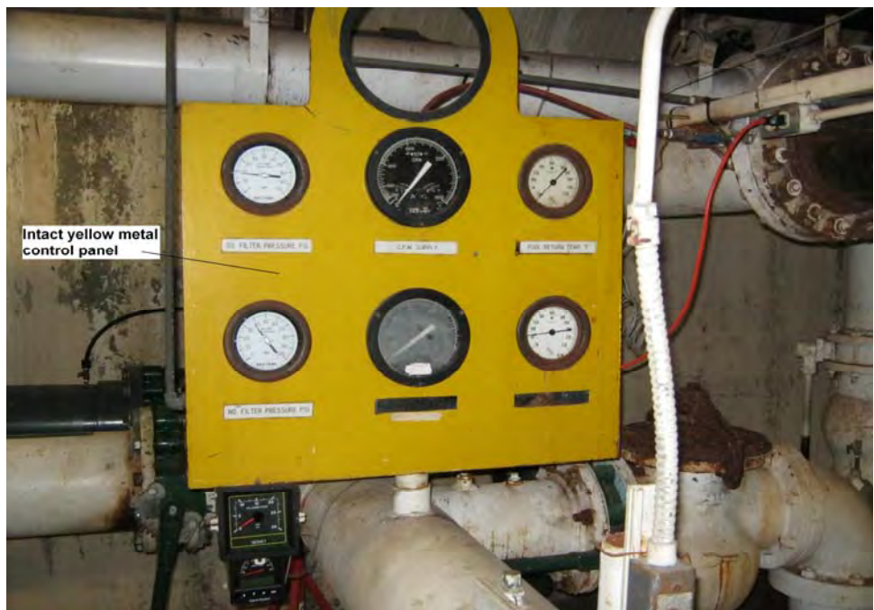
Photograph 24: View of intact lead-containing yellow paint on metal control panel in the filter tank room in the basement of the main pool building.
