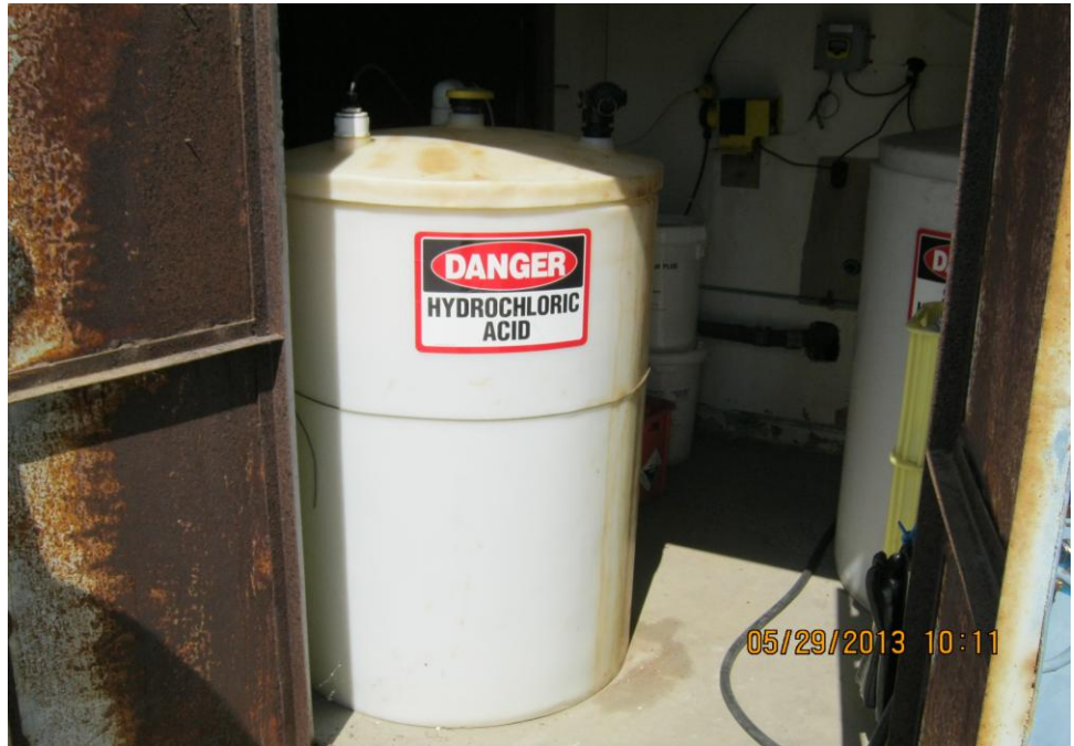
Photograph 5: Looking inside the storage shed at the 150-gallon aboveground storage tanks (ASTs) containing hydrochloric acid and sodium hypochlorite.
