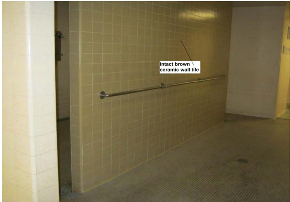
Photograph 31: View of representative intact lead-containing brown ceramic wall tile in the women's, women's executive, men's, men's executive, and men's employee locker rooms in the locker rooms and office building.
