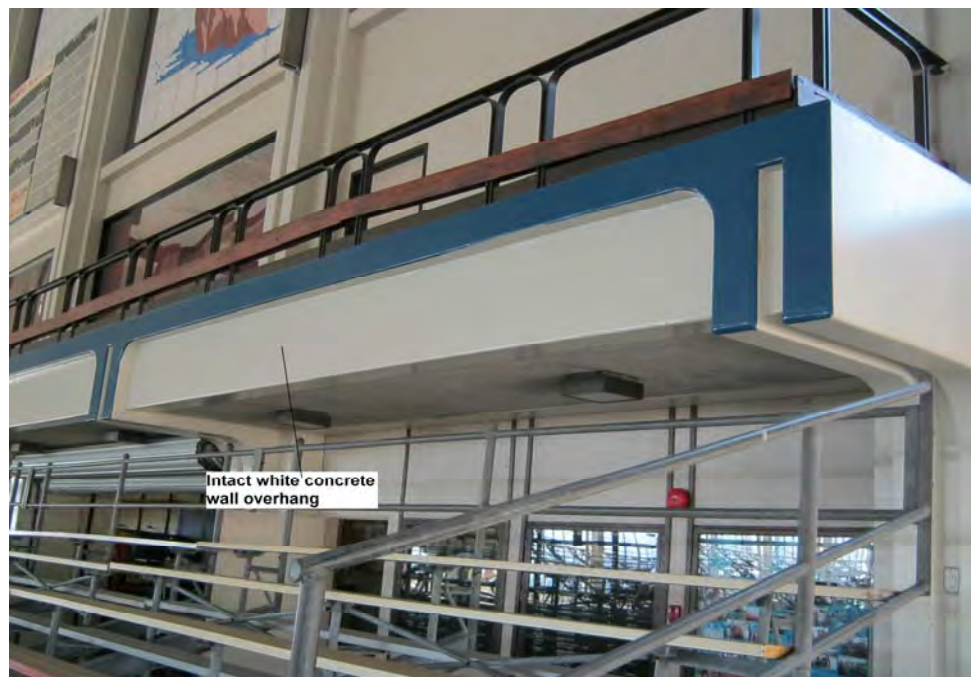
Photograph 20: View of representative intact lead-containing white paint on concrete wall overhang in the main pool building.
