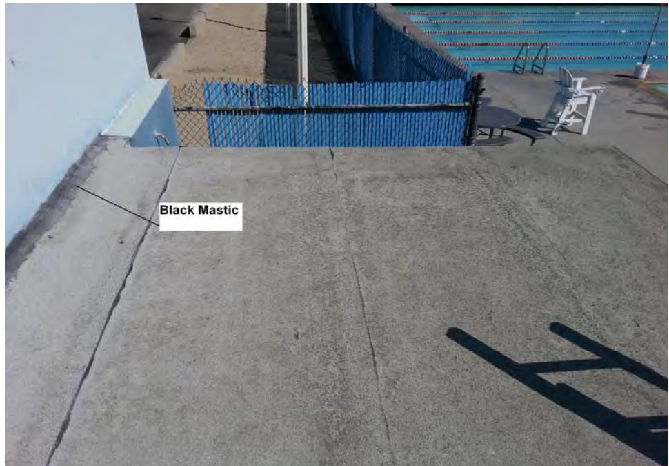
Photograph 11: View of old pool storage building roofing with asbestos containing black mastic.
