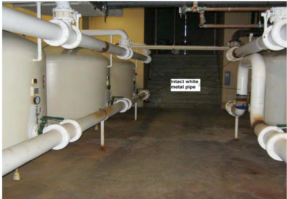
Photograph 23: View of representative intact lead-containing white paint on metal pipes in the filter tank room in the basement of the main pool building.
