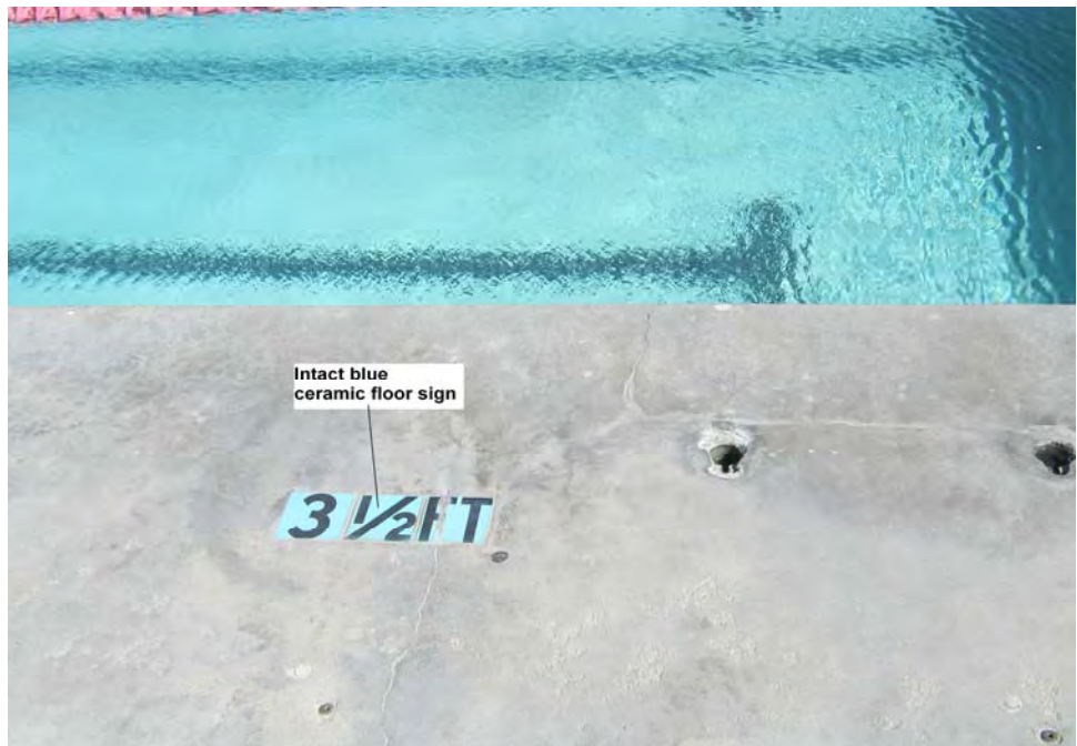
Photograph 32: View of intact lead-containing blue ceramic floor tile in the old pool area.
