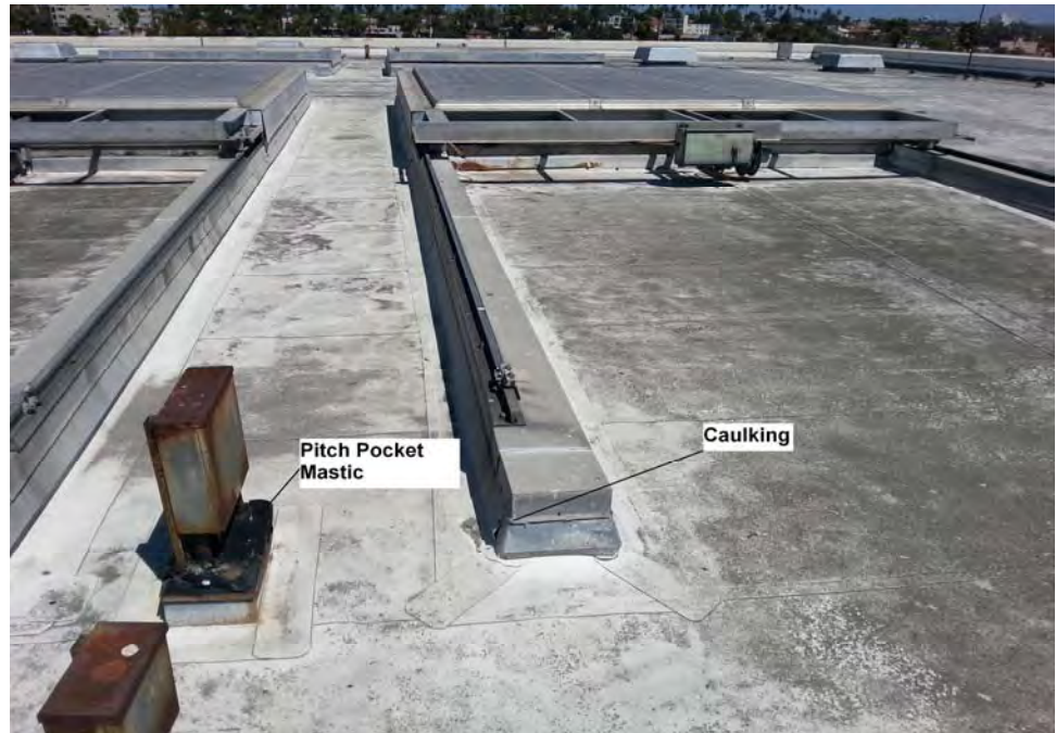
Photograph 3: View of main pool building roofing with asbestos containing materials including penetration mastic and skylight beige caulking.
