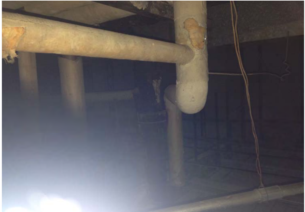
Photograph 7: View of representative asbestos containing cloth-wrapped elbow insulation in the ceiling plenum above the first floor women's restroom within the restaurant building.
