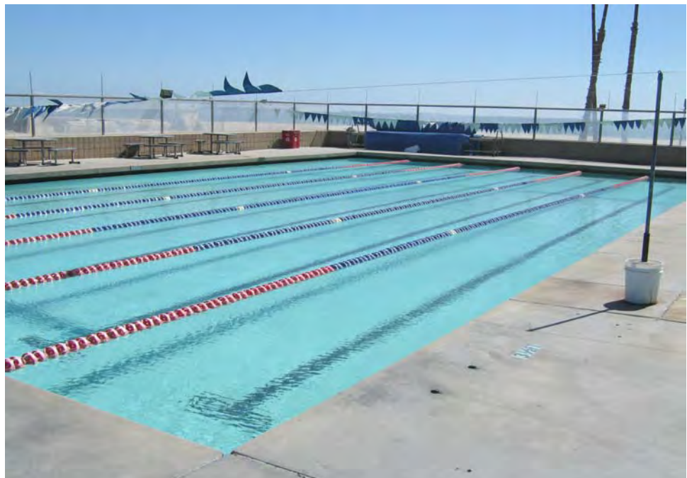
Photograph 34: View of assumed intact lead-containing blue ceramic wall and floor tile and white paint on concrete walls and floor in the swimming pool of the old pool area.
