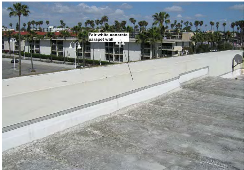
Photograph 12: View of fair lead-containing white paint on parapet concrete wall on the roof of the restaurant building.
