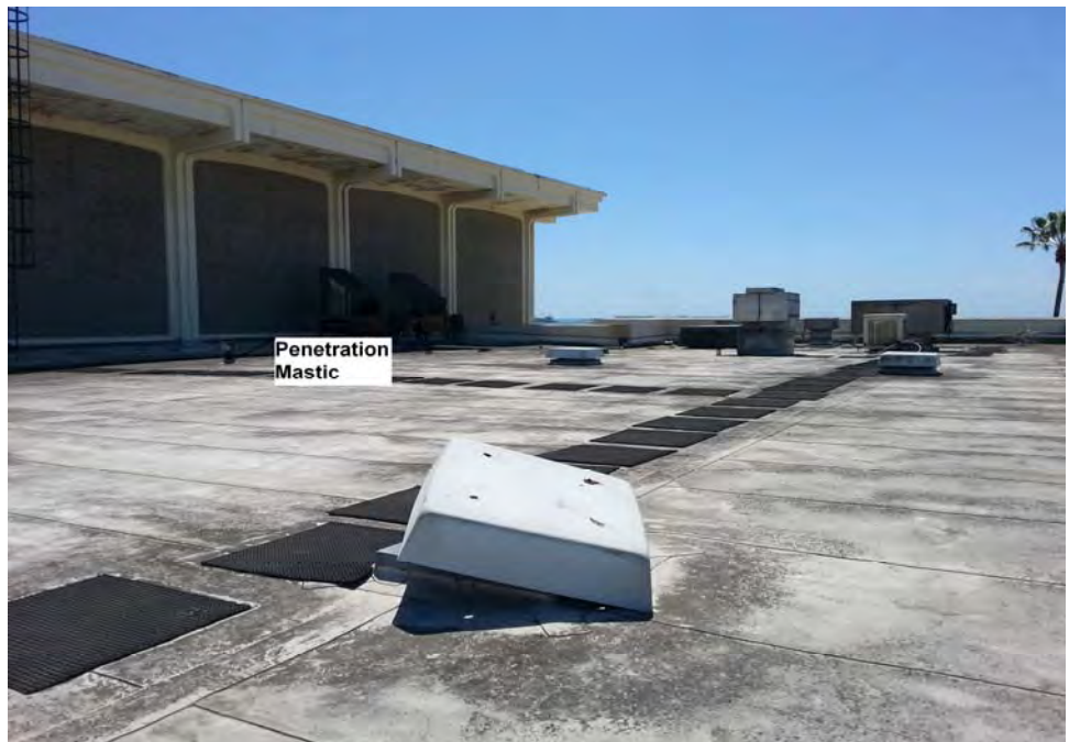
Photograph 6: View of restaurant roofing with asbestos containing penetration mastic.
