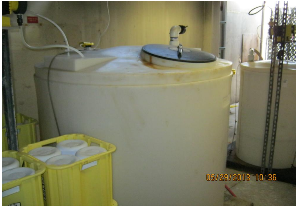
Photograph 11: Looking at the hydrochloric acid and sodium hypochlorite tanks located within the indoor olympic-size pool area.
