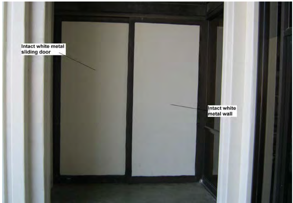
Photograph 26: View of representative intact lead-containing white paint on metal wall and sliding door on the exterior of the locker rooms and office building.
