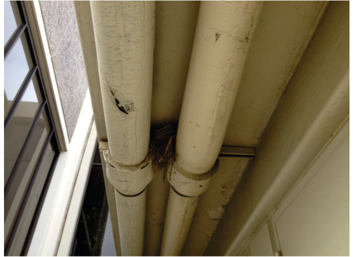
2. Two nests observed on top of pipes that run under Del Mar Room ramp.
