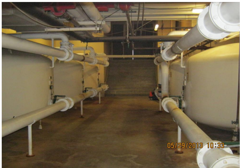
Photograph 10: Looking inside the filter located at the western portion of the indoor olympic-size pool area.
