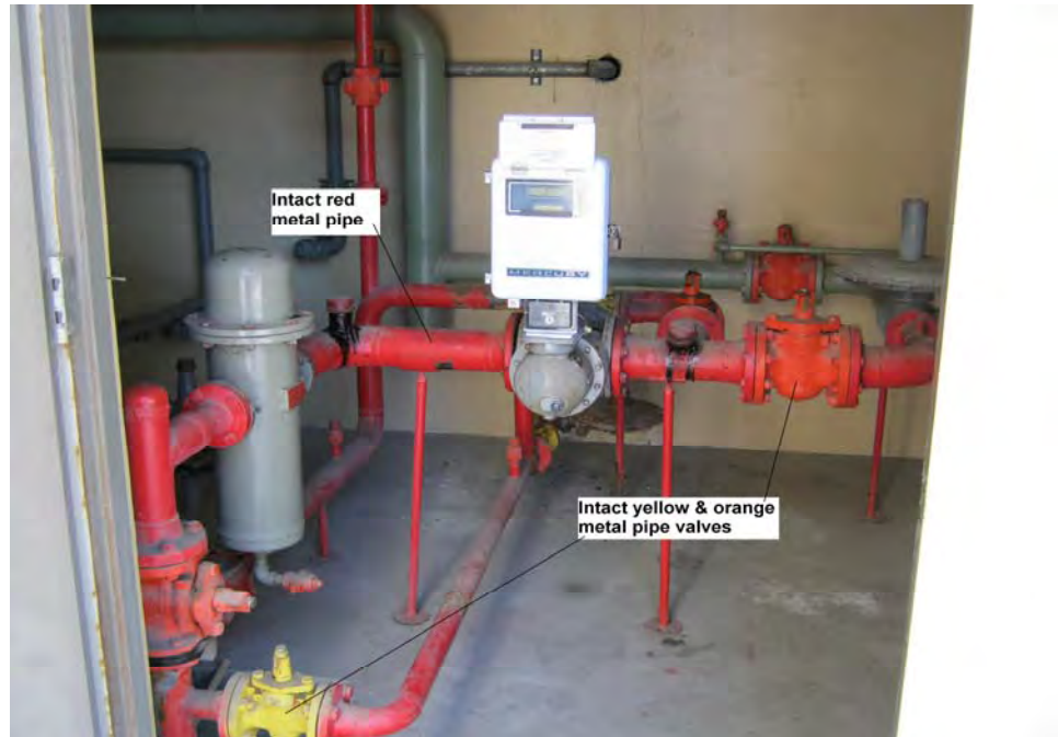
Photograph 17: View of intact lead-containing red paint on metal pipes and yellow and orange paint on metal pipe valves in Room 2 under the ramp.
