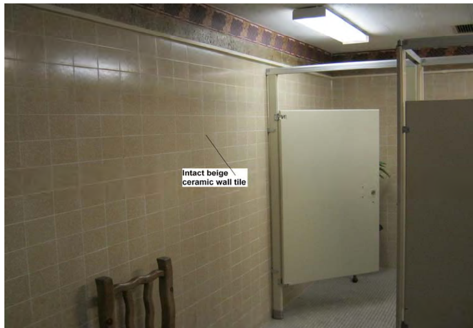
Photograph 14: View of intact lead-containing beige ceramic wall tile in the 2 nd floor men's restroom of the restaurant building.
