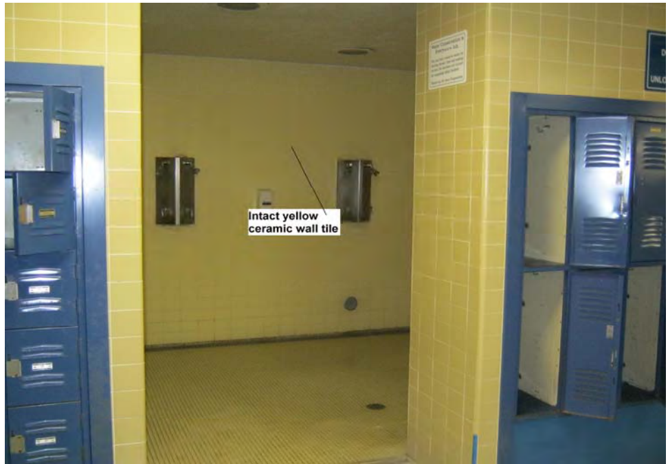
Photograph 27: View of representative intact lead-containing yellow ceramic wall tile in the women's, women's executive, and men's executive locker rooms in the locker rooms and office building.
