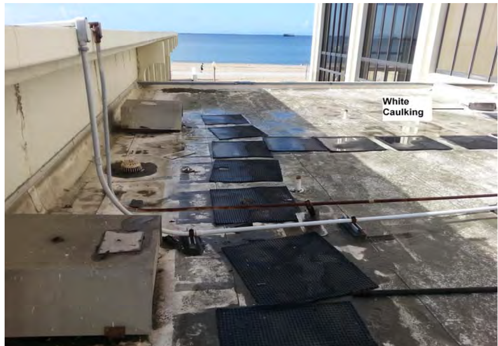
Photograph 4: View of walkway roofing between locker rooms and office building and main pool building with asbestos containing white caulking.
