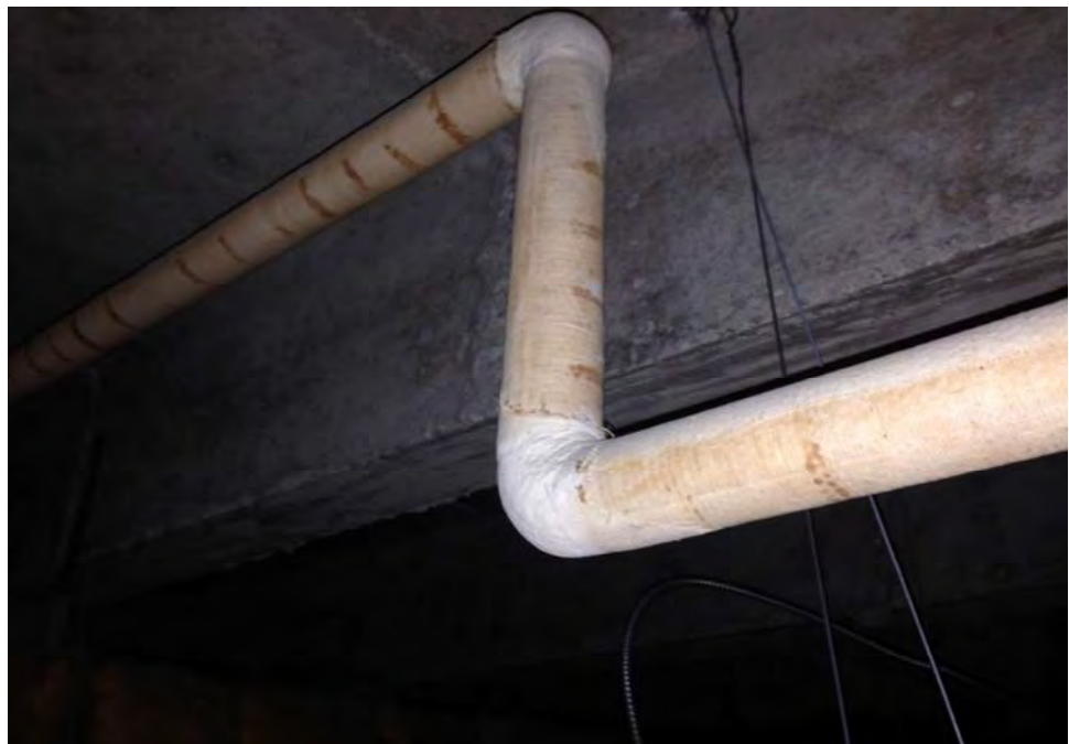
Photograph 2: View of representative asbestos containing cloth-wrapped elbow insulation in the ceiling plenum above the women's locker room in the locker rooms and office building.
