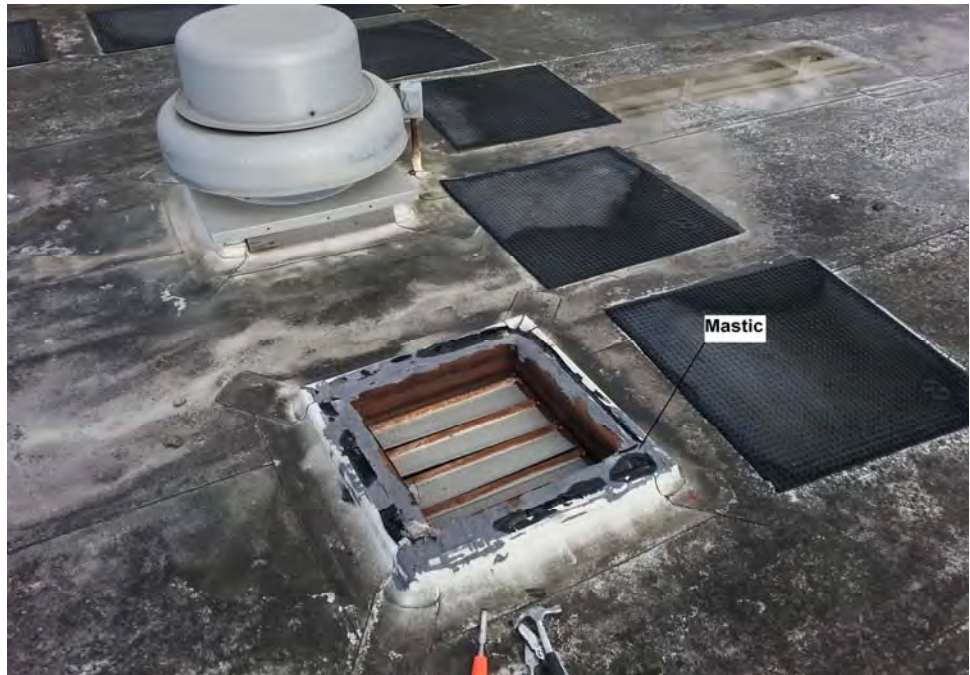
Photograph 1: View of locker rooms and office building roofing with asbestos containing vent penetration mastic.
