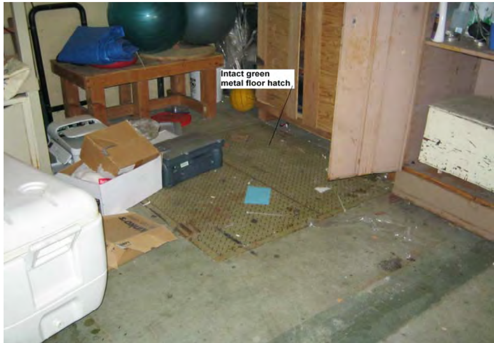
Photograph 21: View of intact lead-containing green paint on metal floor hatch in the storage area of the main pool building.
