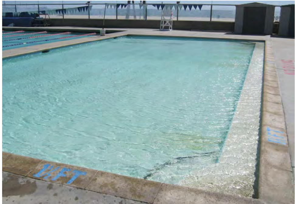
Photograph 33: View of assumed intact lead-containing blue ceramic wall tile and white paint on concrete walls and floor in the wading pool of the old pool area.
